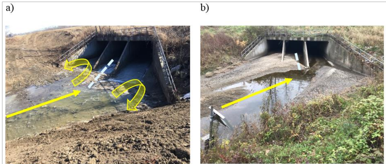
Figure 2.5 Accumulation of sedimentation during eight months of culvert operation from a total cleanup: a) culvert after cleanup in February, 2018; b) sediment deposits in October, 2018. The fine suspension deposits become quickly vegetated retaining sediment at accelerated rates. (Yellow arrow: streamflow dominant direction; dotted white line: culvert direction)
