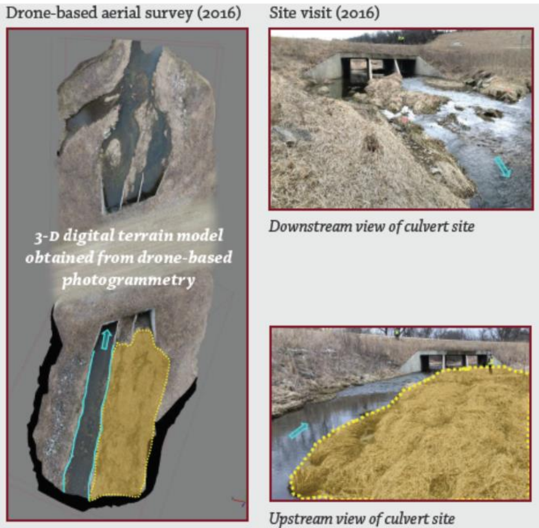
Figure 3.5 Drone-based culvert surveys: a) data acquisition; b) processed data and comparison between aerial- and ground-based photo-documentation
